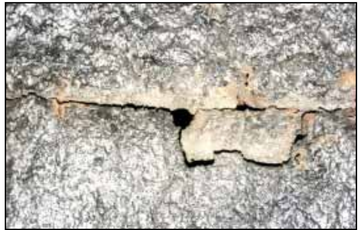
Fig. 15. Corrosion of a RH/OB lining due to air leakage.
