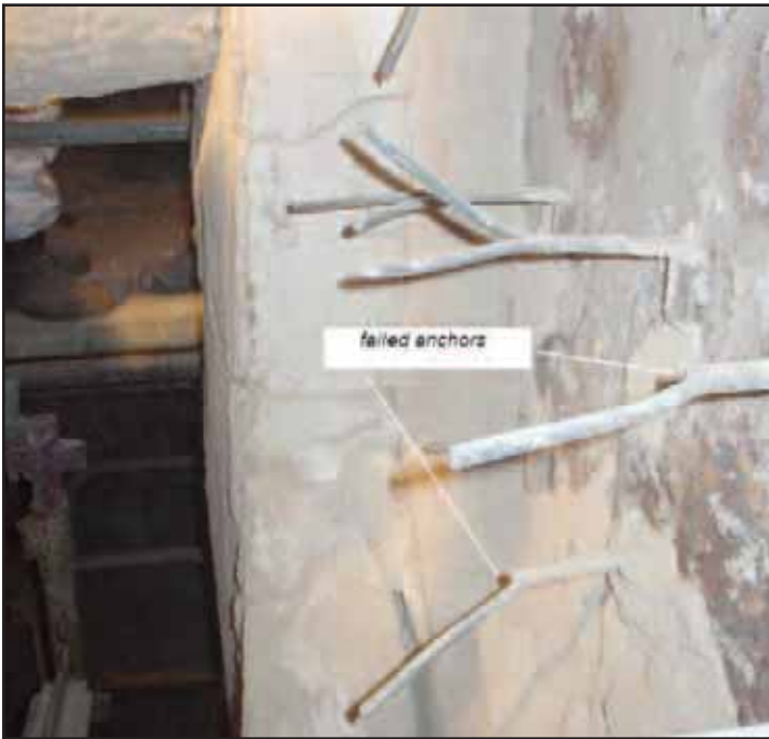
Figure 12. View of failed anchors (10 mm diameter) showing one stem of the vee missing.
