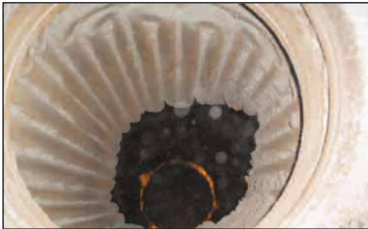
Figure 11. Material reaching the upper part of the brick and ready to set.
