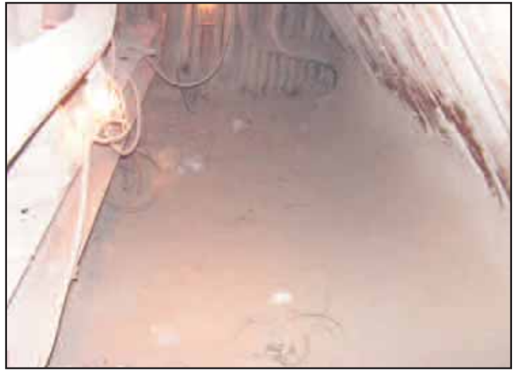
Figure 13. Typical vestibule behind steam drum (note fly ash).
