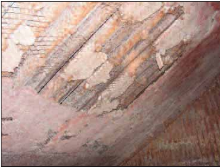
Figure 15. Furnace wall with no expanded metal in some locations.
