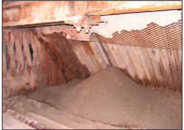
Figure 9. Typical lower furnace vestibule (note how wet the fly is).
