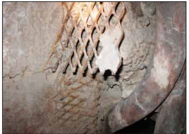
Figure 6. Typical refractory failure inside a lower furnace vestibule.
