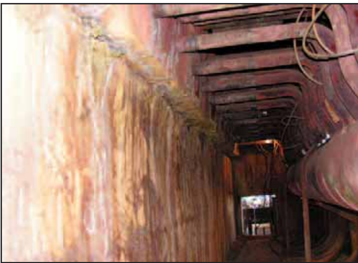
Figure 12. Super heater vestibule (note stain on refractory wall from water washing).
