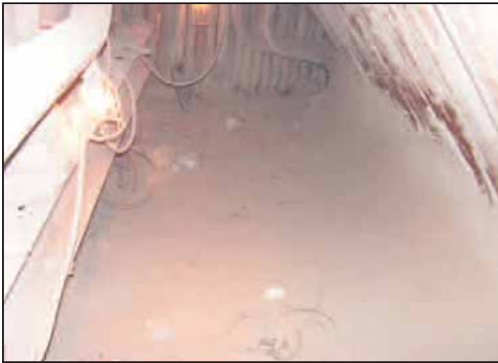
Figure 3. Typical vestibule behind steam drum.
