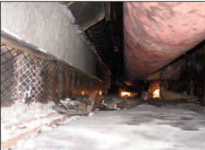
Figure 8. Typical super heater vestibule (note expanded metal on wall).
