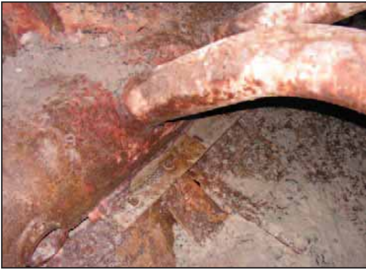
Figure 11. Typical tubes inside a lower vestibule.
