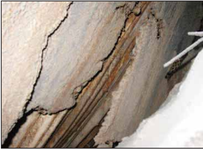
Figure 7. Typical refractory failure inside a lower furnace vestibule.
